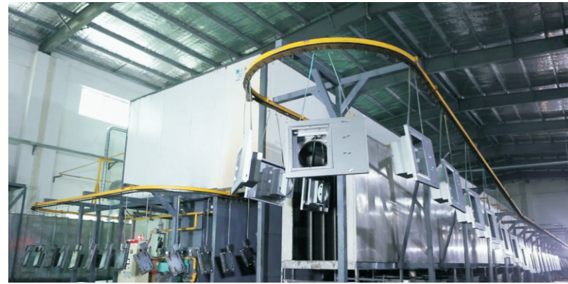
烤漆车间 / Painting Workshop
